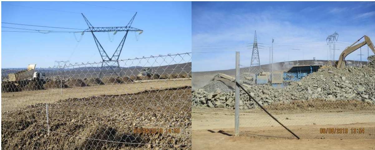
Photo: Layer works at section A (132kV terrace). Photo: Crushing of materials at section D.
