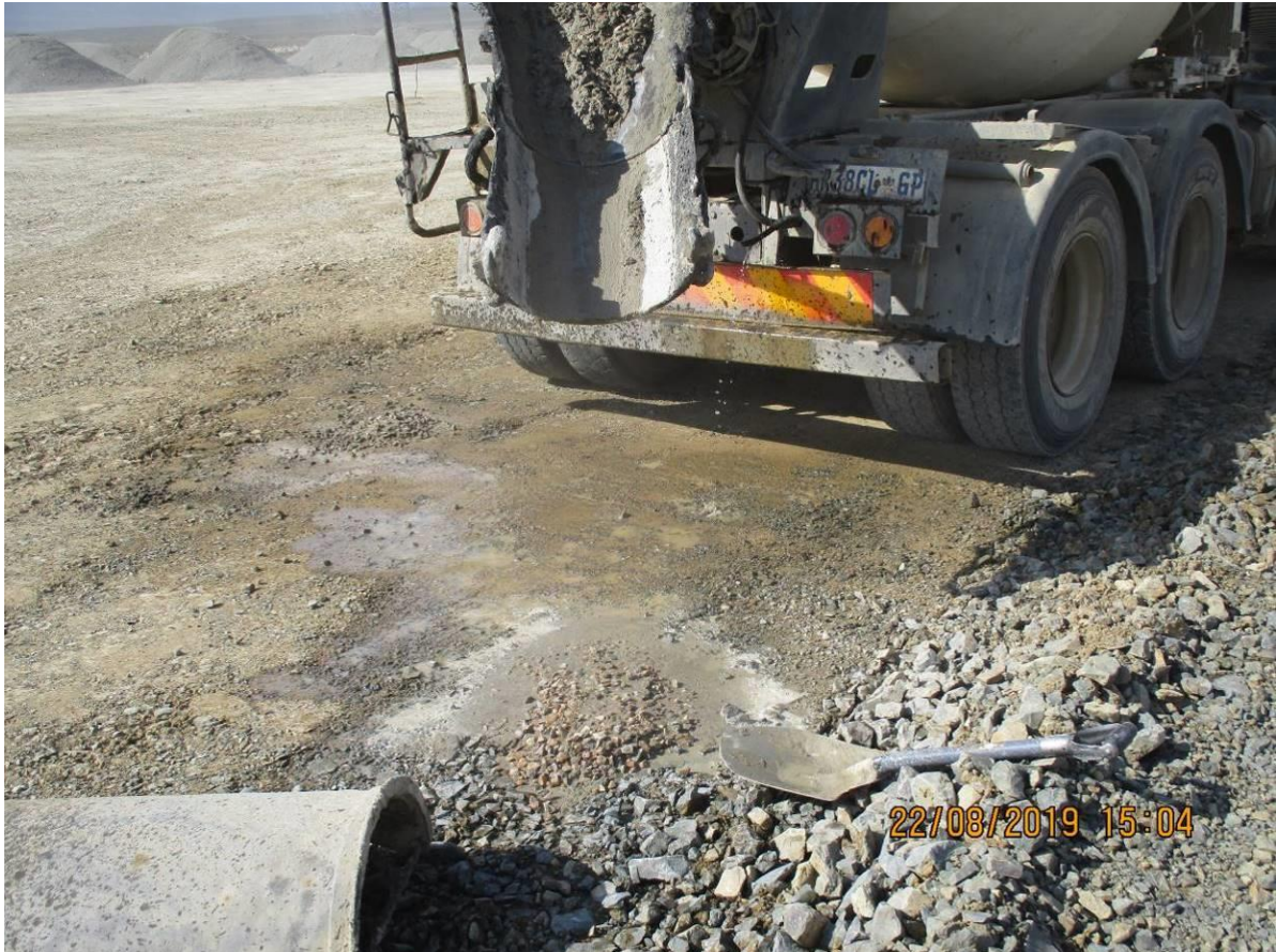
Photo: Concrete spill from mixer truck (Operator washed access concrete on the terrace).
